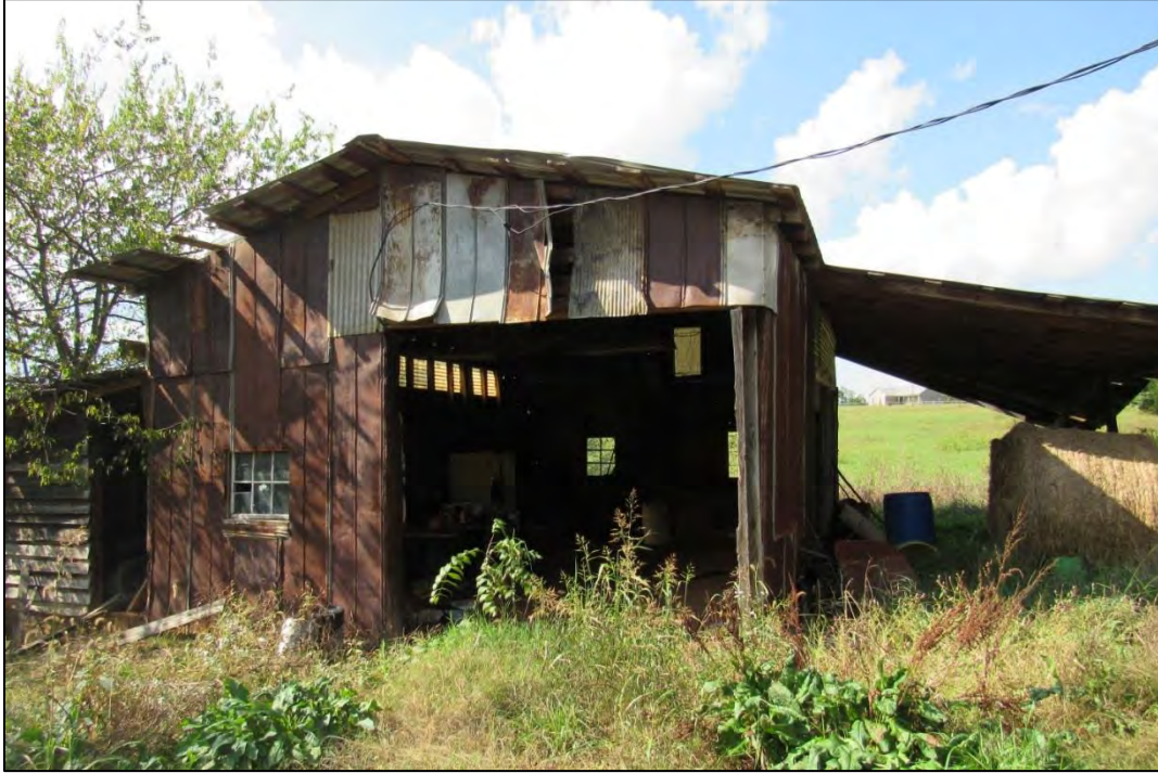
Photo 23: View of Southeast Elevation of Workshop with Lean-to Additions at Either Side
