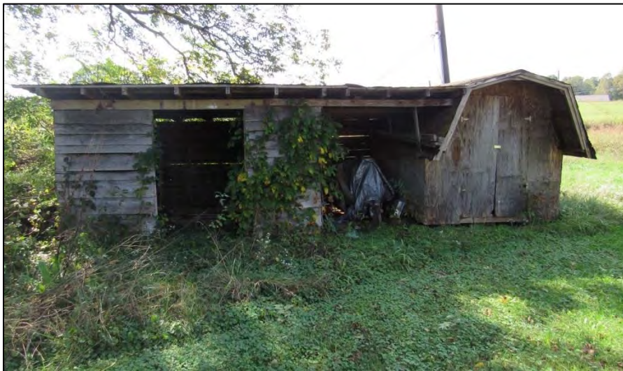
Photo 21: East Elevation of Storage Shed. The circa-1970 shed section is on the left and the circa-1990 section is on the right.
